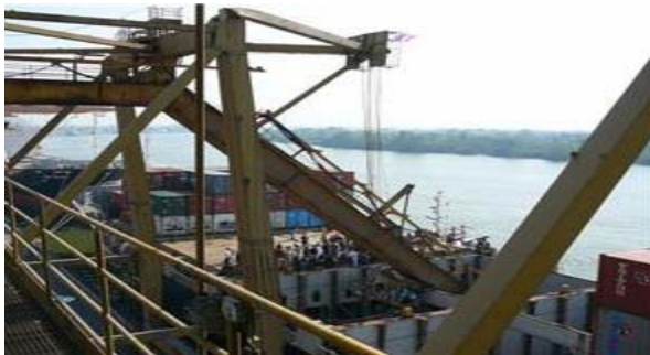
Crane Accident at Bangkok Port terminal
